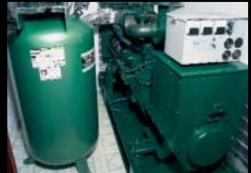
Optional Installed Generator, Air Compressor & A.C.
