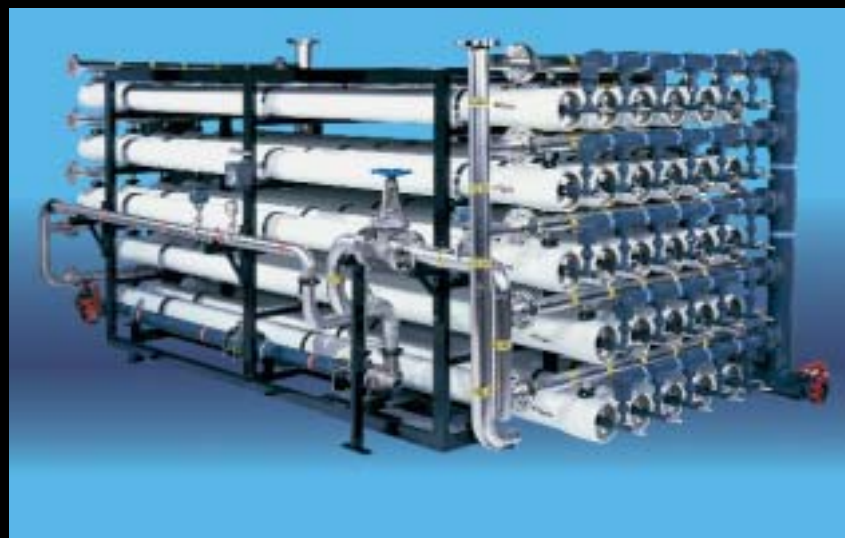
Membranes & Stainless Steel Piping
