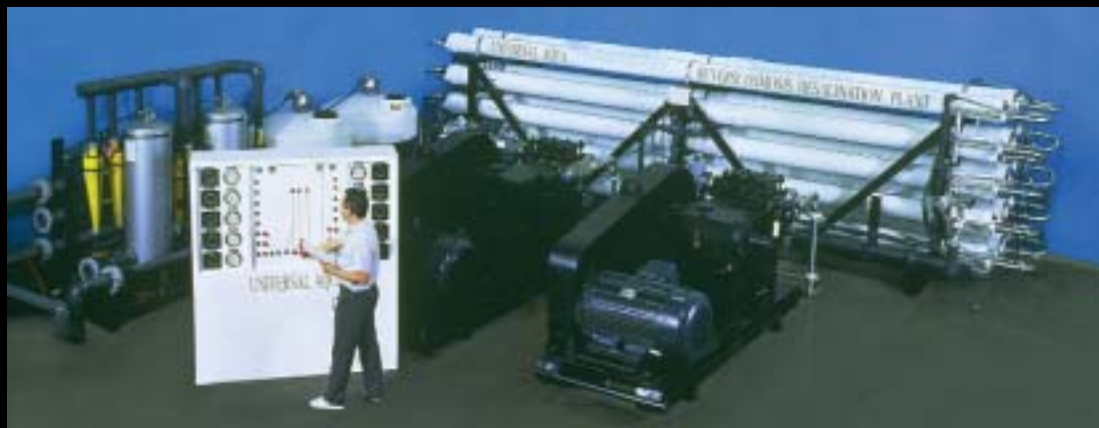
265,000 GPD Desalination Plant
